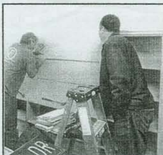
Mark Weinberger, fireplace project manager, observes the removing of bookshelves in the Gillespie Room.
